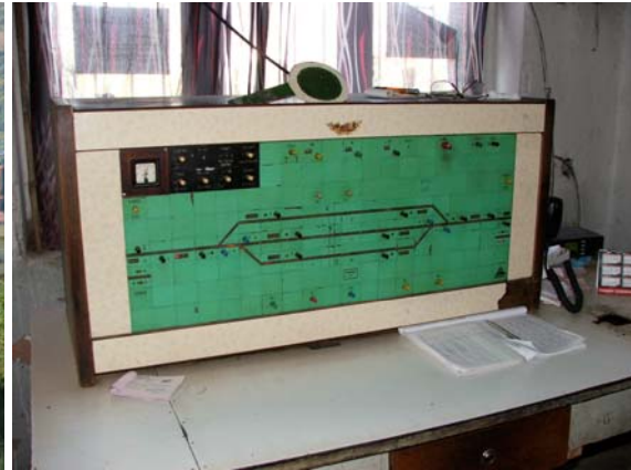
The NX panel and radio equipment at Kavajë.
